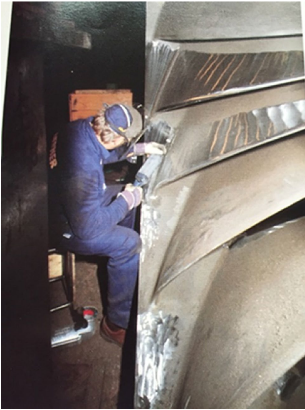
Fig. 1 In this image from 1994, a worker is polishing the surface of a turbine wheel
