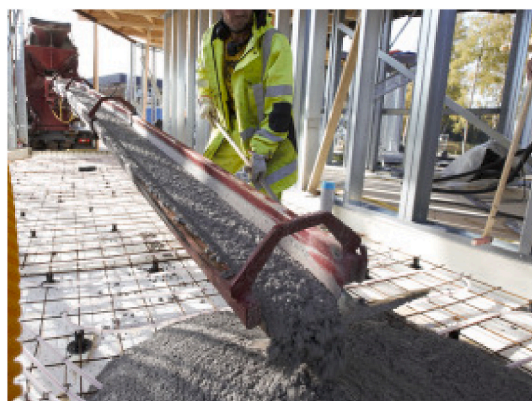
Fig. 12. Casting of an alkali-activated blast furnace slag concrete floor in Lohja, Finland, in 2020 [137].
