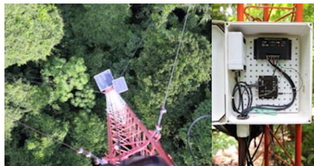
FIGURE 2 The solar panels (left) and electronic equipment (right) used to support individual cameras in the video network. The panels collectively provided up to 90 W of power to recharge a deep-cycle 12-V battery (not shown) during the day, while also powering the camera, GPS antenna, text overlay unit, and DVR. These latter components were then powered by the battery through the night
