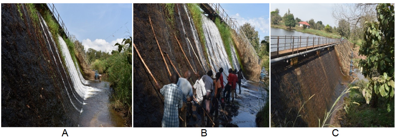
Figure 1. (A) Before “slash and clear” in November 2019, (B) during “slash and clear” at the Maridi dam spillway, and (C) post-“slash and clear” at the Maridi dam, December 2019.
