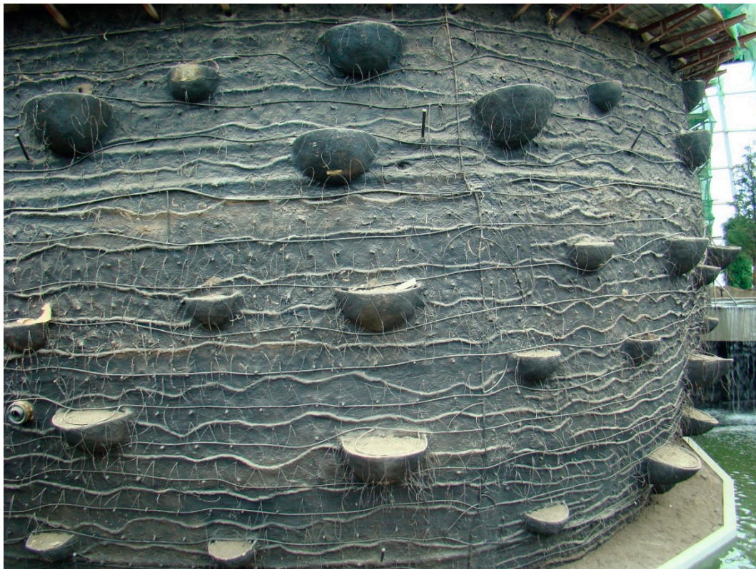
Figure 2. The basic structure of the living wall. The structure is a block building with a mixture of concrete, clay, and organic material (peat) applied as 2 inches of thick slurry over a wire mesh attached to the exterior. The pop-out baskets are designed to provide space for the soil and root.
