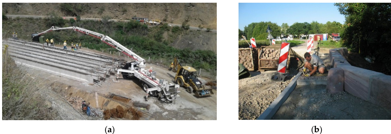
Figure 3. Photographs of construction sites and workers in Colombia while working on bridge construction (a) and in Germany while paving a walkway (b). The dosimeter is worn on the upper left arm (black strip) without any impairment of the task being carried out. (©SURA, ©IFA).
