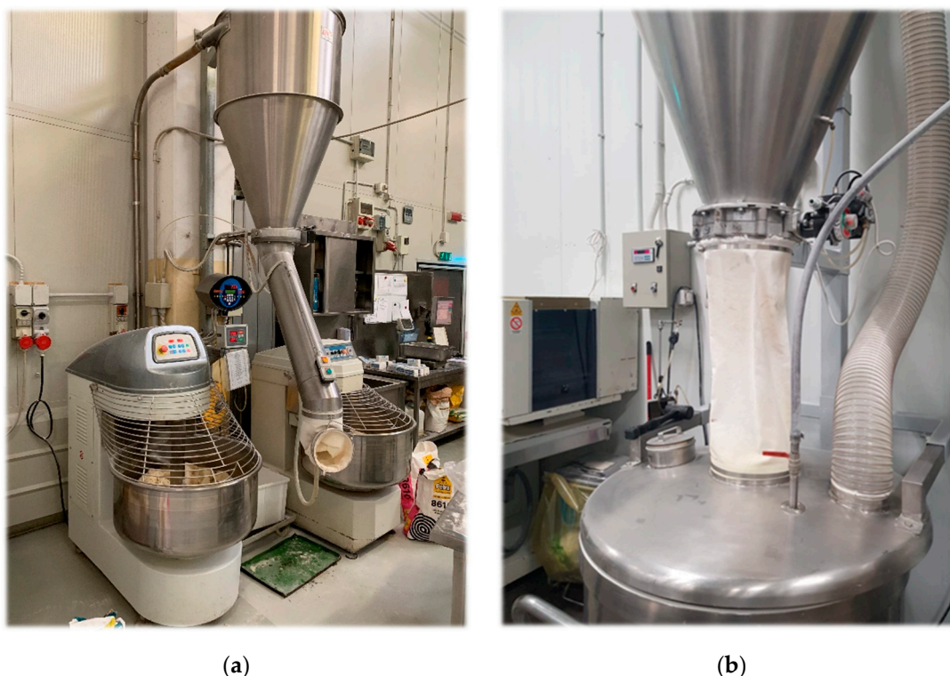
Figure 1. Installation of a sleeve at the end of pipeline (a); installation of a lid and a local exhaust ventilation system on a mixer tub (b).
