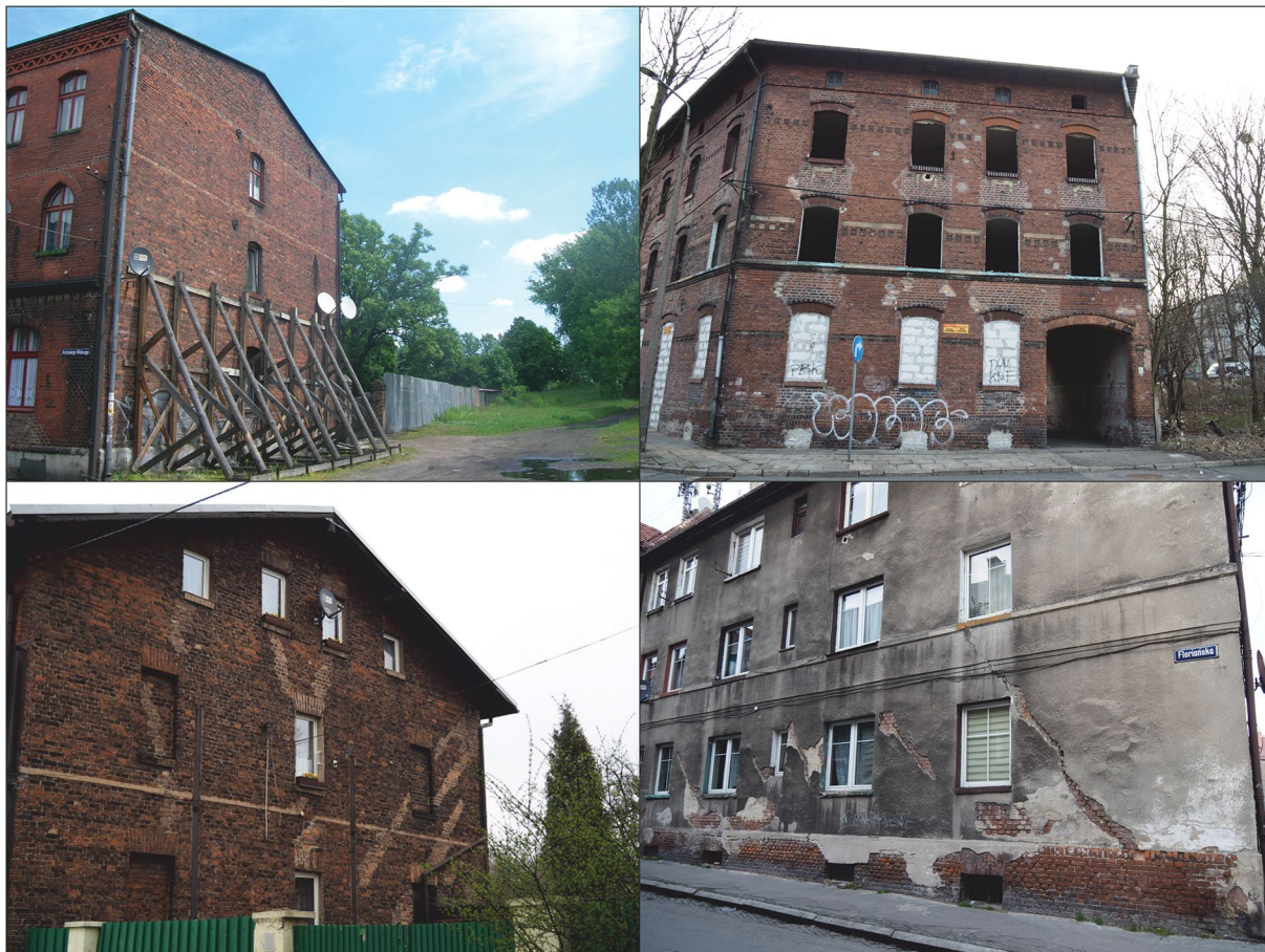
Figure 6. Examples of damage to Bytom's urban fabric as a consequence of land subsidence (photo: M. Solarski).
