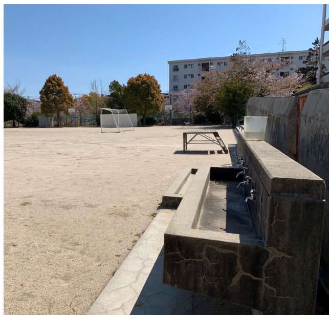
Fig. 1 Water supply facility between the playground and school building.
