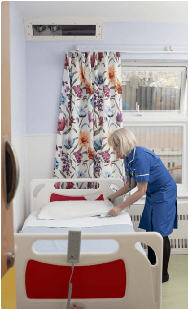
FIGURE 1. The system hardware installed above the bed in a patient room.
