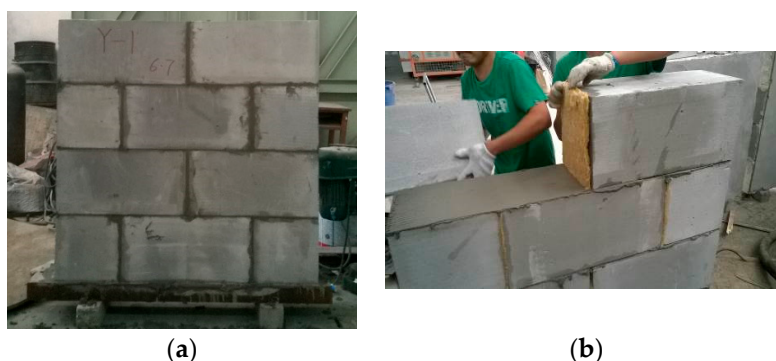
Figure 1. Construction of wall specimens: (a) overview; (b) vertical joints filled with mineral wool plate.
