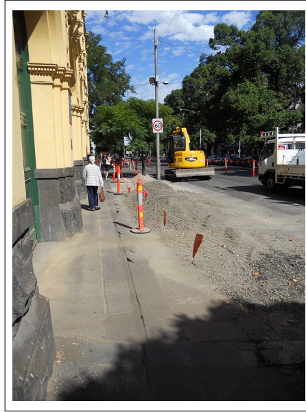
Figure 2. Clear pedestrian footpath barricaded from roadworks in Melbourne. Photograph by Dean Johnson. Used with permission.
