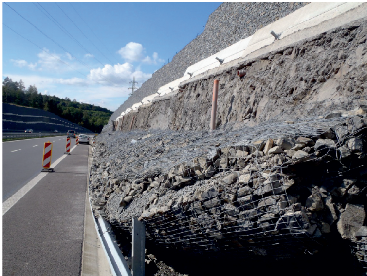
Figure 13. View of the collapsed gabion wall at the given location prior to the installation of the monitoring system.
