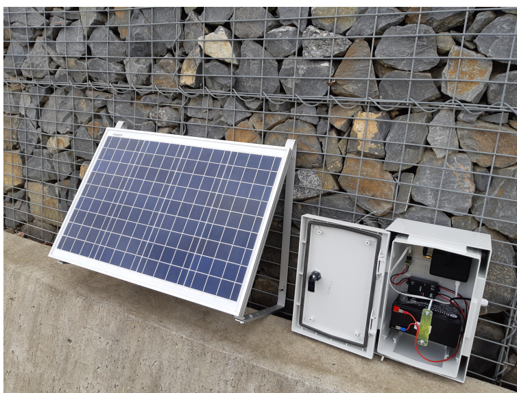
Figure 15. Image of the IQRF ® /GSM gateway and solar panel installed on the gabion wall.
