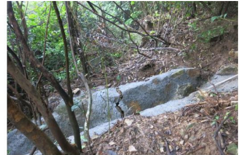
crack in the intercepting ditch for #12 slope
