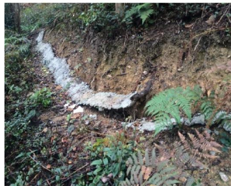
cracks in #10 slope (still active after sealing)
