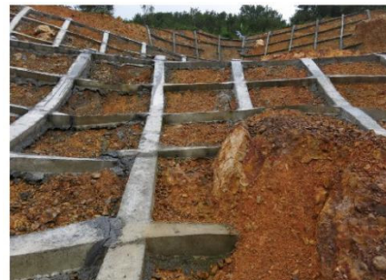
damage of the grille retaining wall
