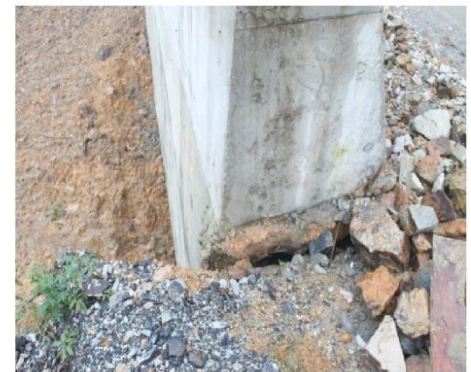
crack in the retaining wall for #12 slope
