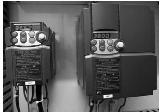
Fig. 5. Inverters I and II
