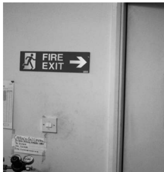
Fig. 16. Fire exit sign
