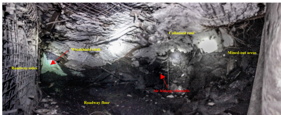
Figure 10. Collapse zone of the lower end of the working face.
