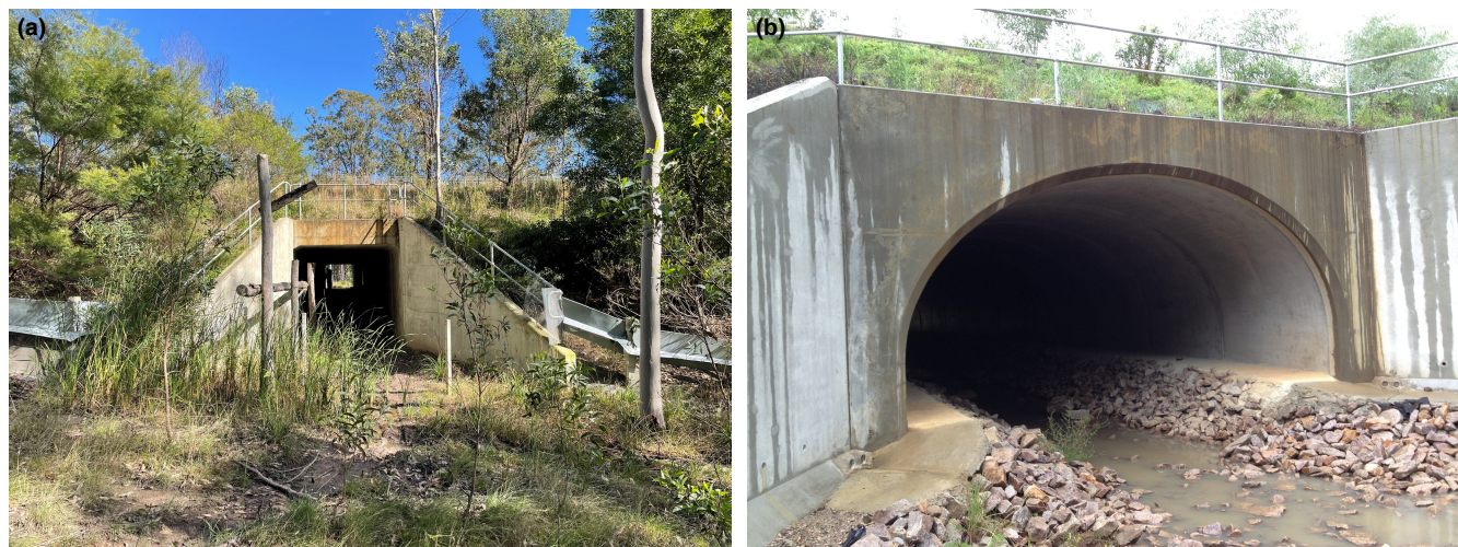
FIGURE 3 Underpasses at Grafton. (a) A fauna underpass with timber railing. (b) The Bebo arch underpass contained a center drainage area and raised passageways on each side
