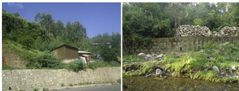
Figure 9. Retaining wall constructed to protect soil subsidence from mountainous areas (a) and river banks (b).
