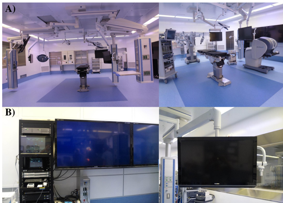
Figure 2 The inside views and equipment of the MISC robotic-operating theater are shown. A) The floor space is 98 m 2 . B) This theater has six fixed monitors and one movable monitor. The six fixed monitors include two sets of 70 inch and four sets of 32 inch-sized monitors. One movable monitor is 46 inch in size. Four sets of 32 inch size fixed monitors and one movable monitor are capable of 3D display.
