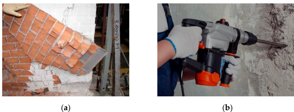
Figure 4. Example of nonreversible retrofit interventions: (a) epoxy-bonded FRP reinforcement is very difficult to be removed, and this causes damage to the masonry material; (b) reinforced concrete jacketing can only be removed with a demolition hammer.
