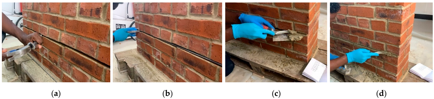
Figure 17. Application phases of titanium alloy threaded rods (bed joint reinforcement): (a) removal of the existing mortar from the bed joint; (b) application of the titanium rod; (c,d) repointing with new mortar [43].
