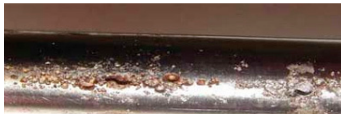
Figure 5. Pitting corrosion on stainless steel [28].
