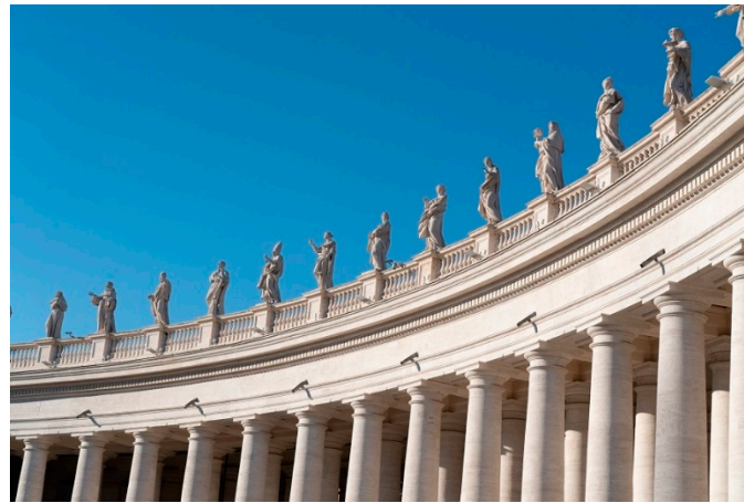
Figure 12. 17th century Bernini statues and colonnades, Vatican City. The marble columns are 16 m in height, and the overlying statues are 3.1 m. Cracking was recently detected in several statues and columns, and titanium reinforcements were used for repair.
