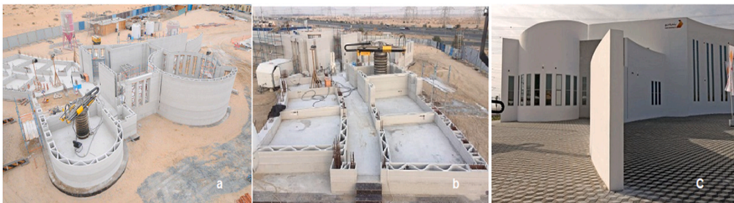
Fig. 7. 3D printed building in Dubai by Apis Cor: a) and b) during printing and C) finished in its environment.
