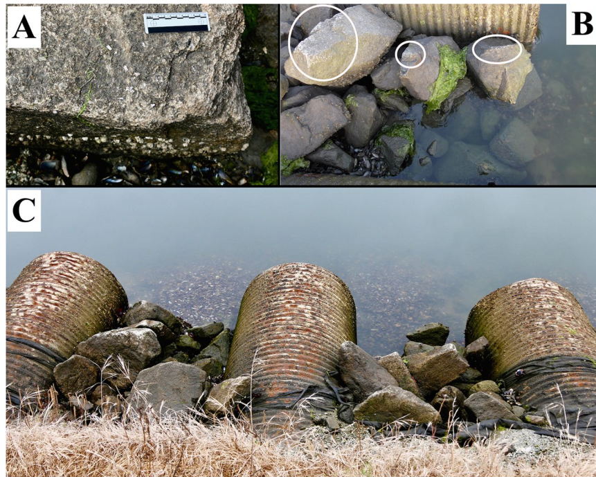
Figure 4. Use-wear damage on rocks at the Bennett Slough Culverts (BSC) site. (A) Sea otter damage on the corner of a quartzite boulder at BSC South; the scale is 10 cm. (B) Emergent boulders damaged by sea otters on their upper surfaces (circled) at BSC North, with the rocks further from the water topographically higher; the water level is mid-height. (C) Emergent anvils at low tide at BSC North, with the boulders seen in (B) on the left. Mussel shell deposits are visible above and below water in the three views.
