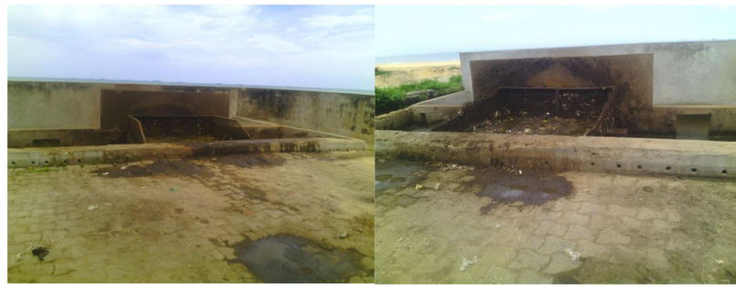
(a) Bar screens at the SIBEAU treatment station
