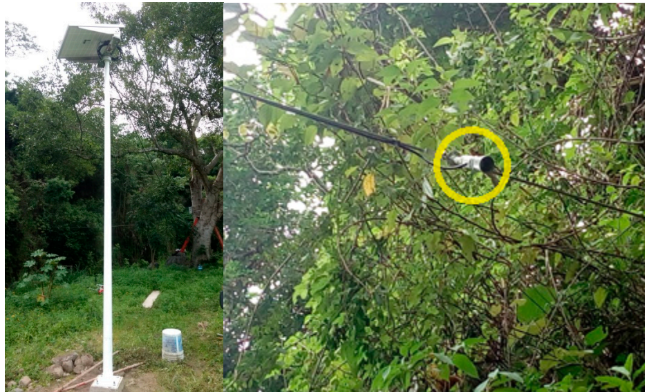
Figure 18. Positioned solar panel and ultrasonic sensor.
