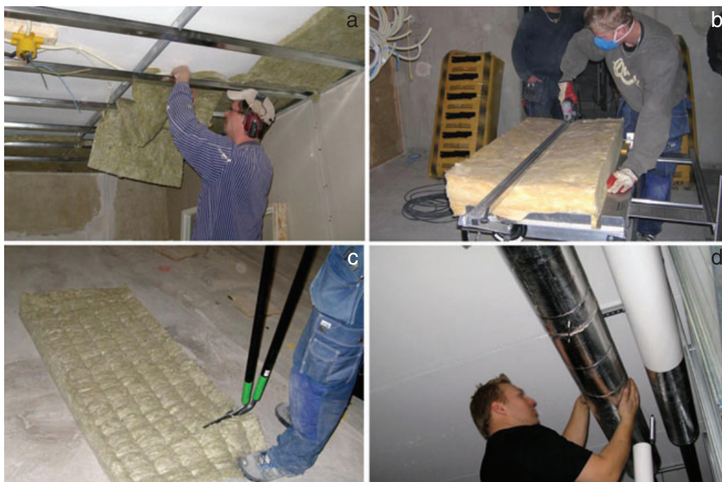
Fig. 1. Some occupational insulation tasks: inner roof insulation (a), cutting a batt for inner room insulation (b), cutting a ventilation insulation batt (c), and installing ventilation pipe insulation (d).
