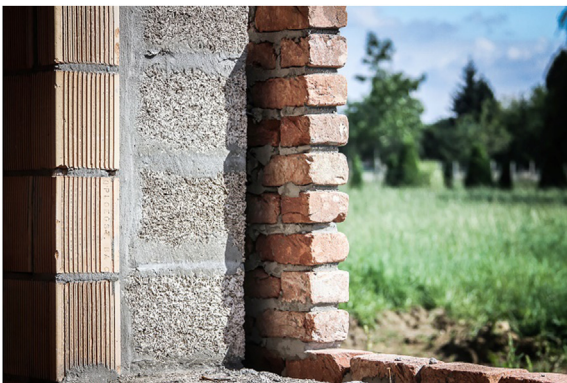
Figure 5. Hempcrete blocks with load bearing blocks [193].
