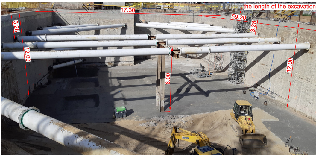
Figure 3. Protection of deep excavation by means of diaphragm wall and struts system.
