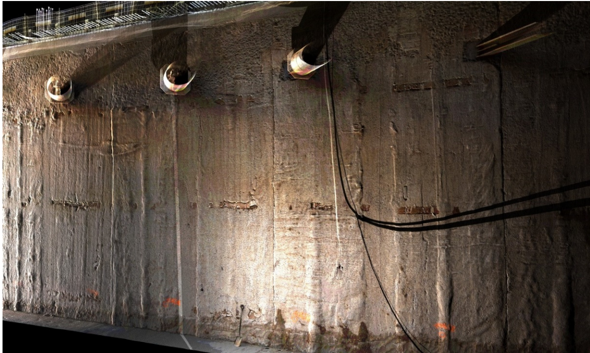
Figure 7. View of the point cloud (in the RGB color space) of northern diaphragm wall.
