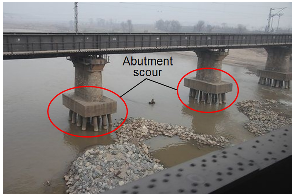
Fig 1. Erosion at the piers of Longhai Railway bridge in Xianyang, China (Modified from the photo in China Construction News [22]).
