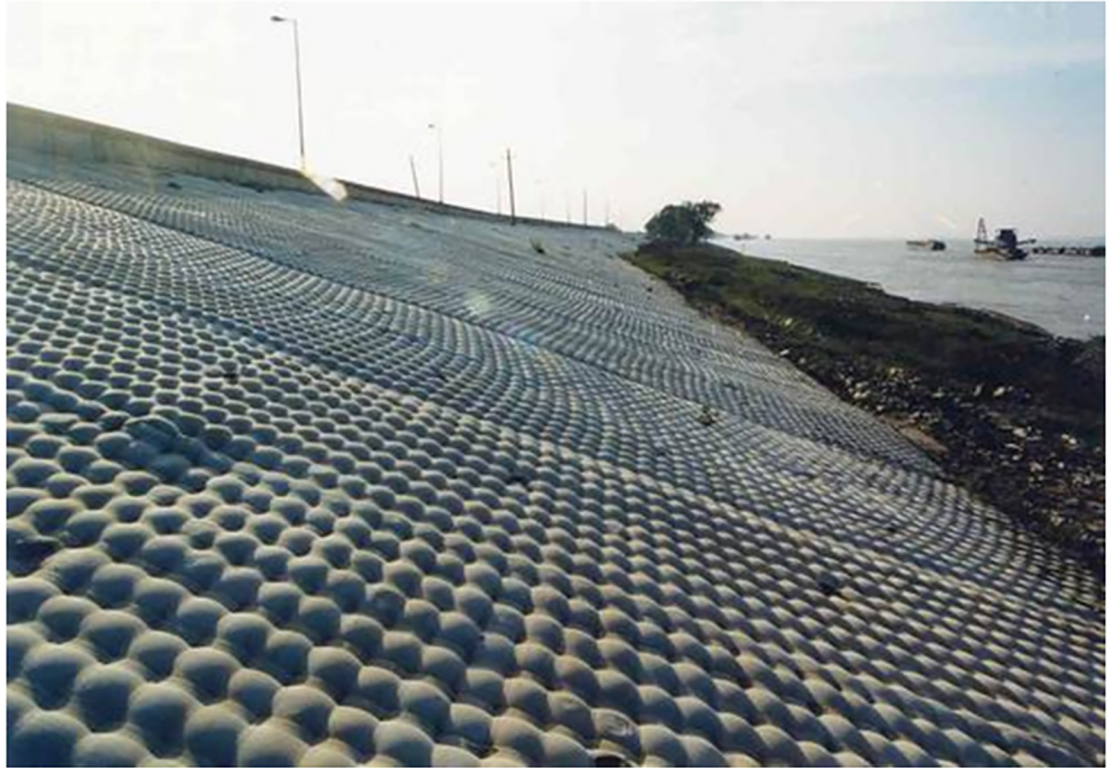
Fig 2. Revetment made of geosynthetic structures on the bank of the Yangtze River in Jiujiang, China.
