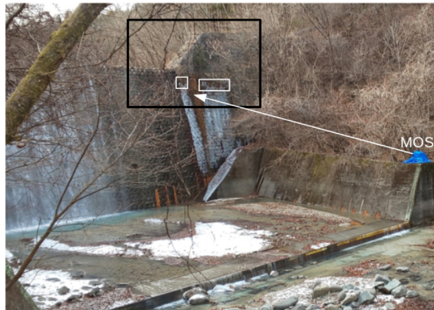
Figure 1. The photograph of the inspected sabo dam in the Karasu River, Gunma, Japan
