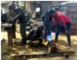
Picture 1: Apprentice learning without protective equipment
