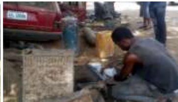
Picture 2: Welder working without protective goggle
