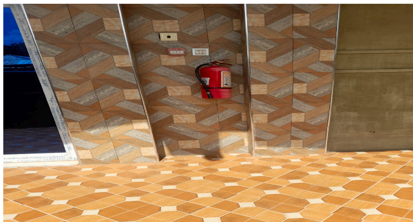
Fig. 4. A fire extinguisher at business premises near a fuel station.
