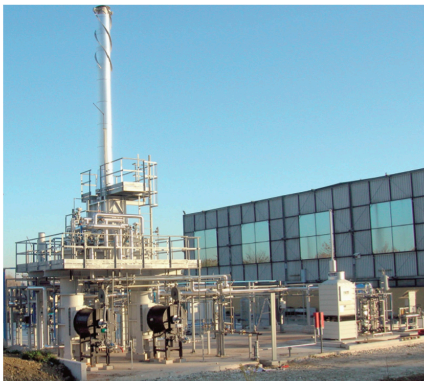
Figure 1. Overall view of the Pilot Plant [21].
