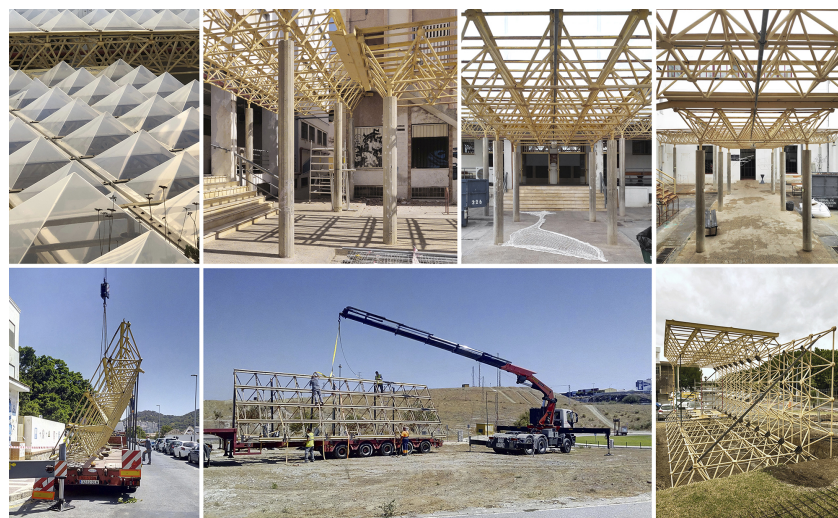
Figure 2. Images of the construction process of the Smart Tree. The top row shows the previous state of the structures located in the courtyard of the Faculty of Fine Arts. The bottom row shows the process of moving and assembling the recycled structures next to the Faculty of Science.
