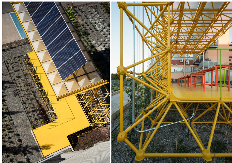
Figure 6. (Left): photovoltaic panels attached to the pavilion structure. (Right): the sensor connection ducts attached to the pavilion structure.
