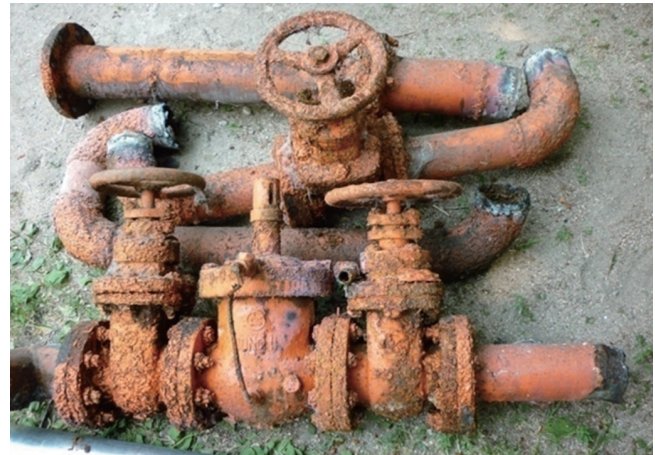
Fig. 4. The corroded water pipes in the apartment complex, Seoul, Korea.
