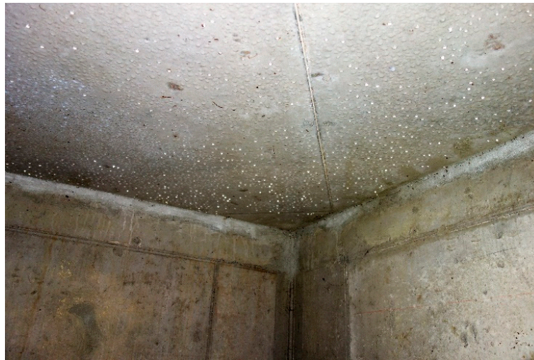
Figure 18. Condensation on the bottom side of the roof slab when the inspection pit and the connecting drainage pipes are operational.
