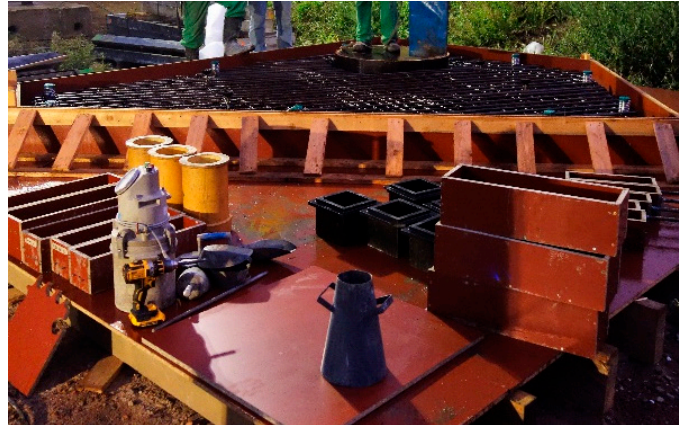
Figure 1. Formwork of the roof slab with the molds of the accompanying lab specimens in front.
