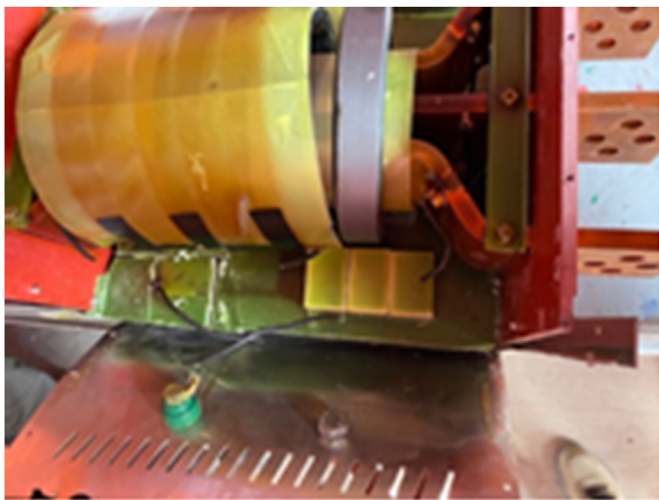
Figure 16. AC filter explosion.
