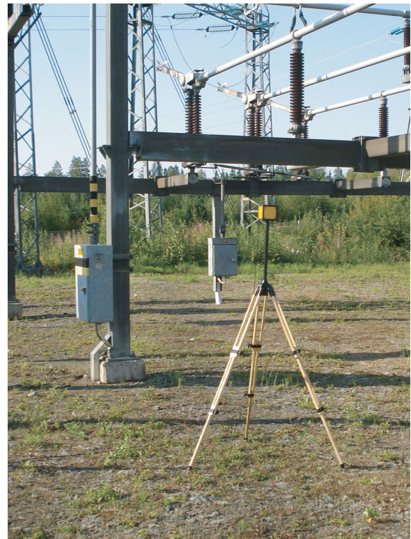
Figure 1. Example of electric field measurement at a 110 kV substation.
