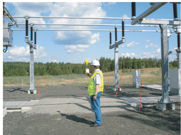
Figure 2. Example of magnetic field measurement at a 110 kV substation.
