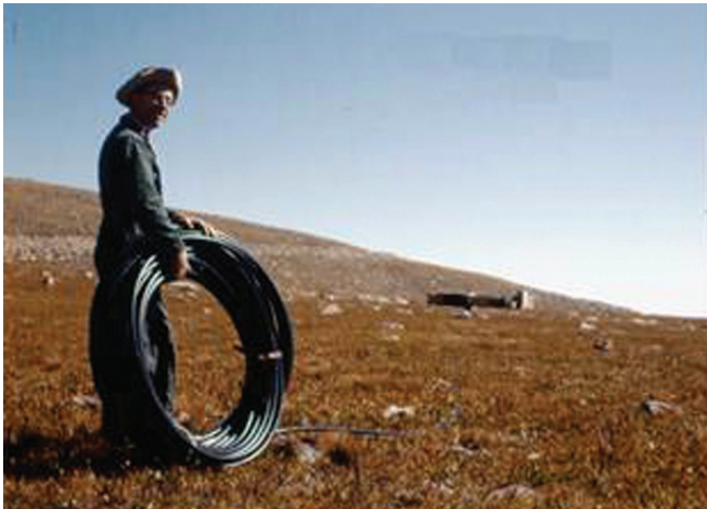
Figure 2: Bob laying out 1,200 feet of flexible pipe to siphon fresh water from Summit Lake to the water troughs in the corral.
