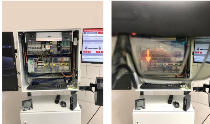
Figure 5. Actual view of a control cabinet; left side: control cabinet seen without the glasses; right side: control cabinet as seen through the right lens of the AR glasses, with virtual red arrow visible (the top grey field is the glasses frame and to the left one can see the glasses bridge and nose pads). Photographs: Szajna A.
