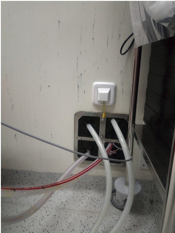
FIG. 2. Tubes passing through hole in the wall, inside the operating room.
