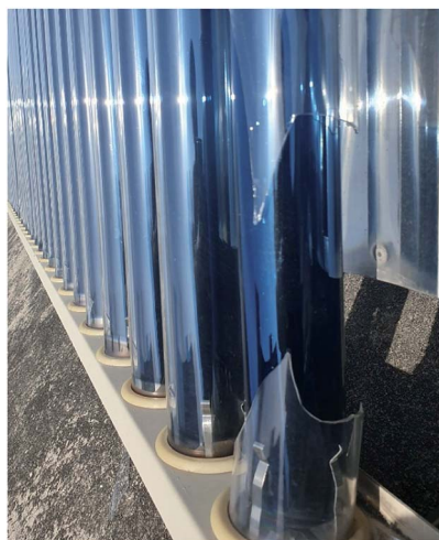
Fig. 1 Double glass tubes of ETC damaged by the impact of a small object flying in a strong wind.
