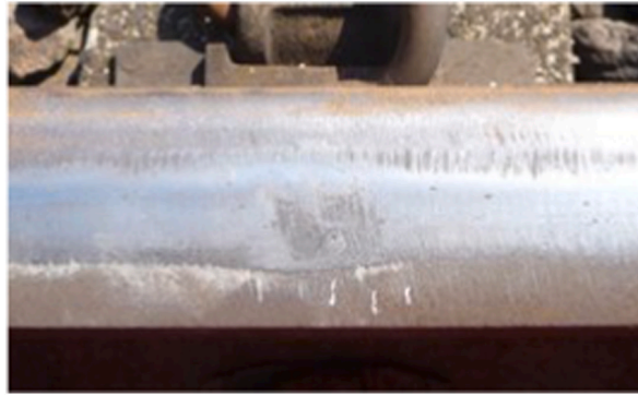
Fig. 1. Example squat defect [authors own photograph].
