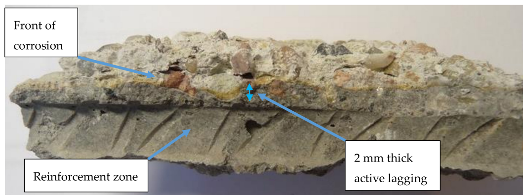
Figure 7. Thickness of non-corroded lagging in borehole No. 1 is only 2 mm.
