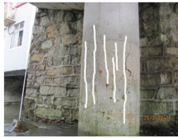
Figure 5. Cracks on The surface of pier #1.
