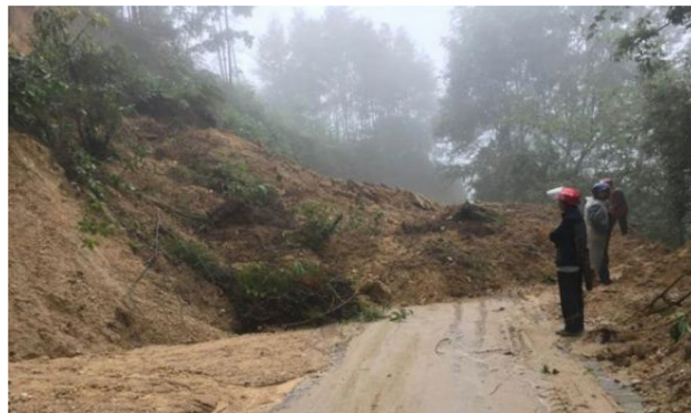
Figure 1. Mountain landslide blocking road.
