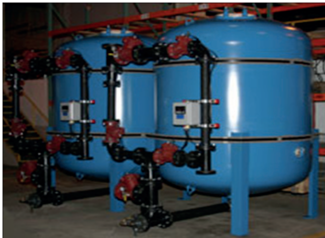
Figure 2: Uranium removal from drinking water
