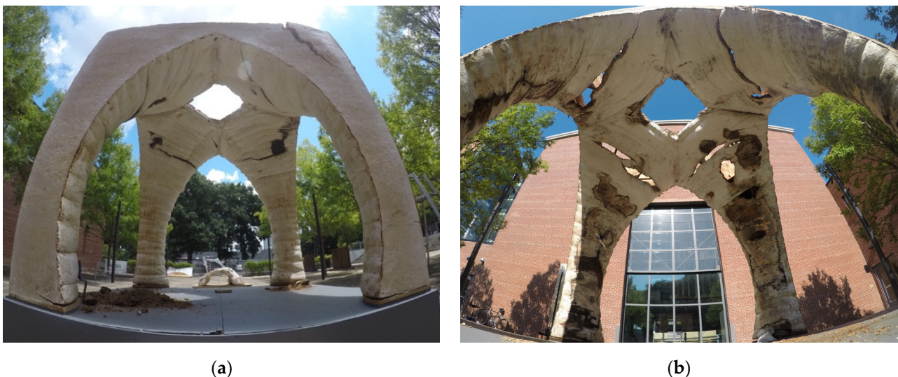
Figure 3. Decay of the Monolito Micelio. (a) Cracking and decay of the structure after three months caused by expansion and contraction of the material matrix against the internal reinforcing structure; (b) cracking, decay, and infestation of the structure after four months. Photos by the author.
