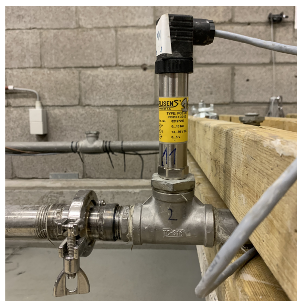
Figure 6. Example of a pressure sensor being screwed in a T-connector as close as possible to the virtual pipe wall.
