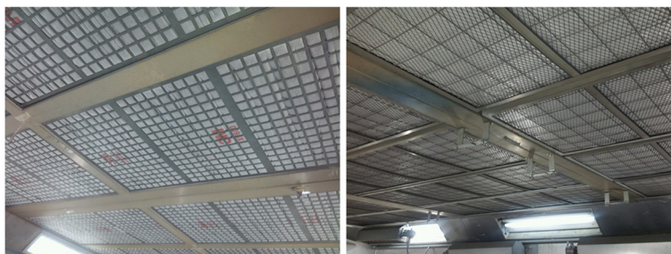
Figure 5 Ceiling inlet in the painting booth.
