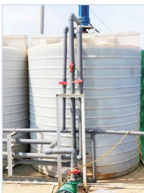
Fig. 6 Chemical solution tank.
